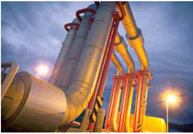
Petrochemical and Refining
